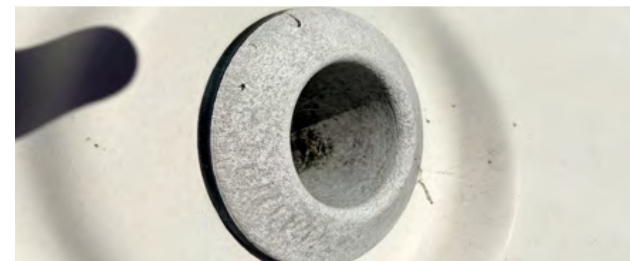
A very brittle and UV-damaged skin fitting long overdue for replacement. It is a potential source for down flooding. Defective items such as this should be identified from both deck inspections and 10-year haul-out refit.
