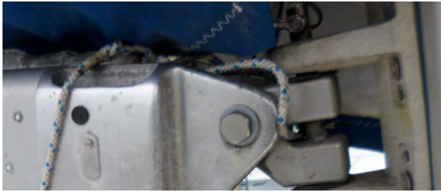
A gooseneck fitting on a sailing catamaran mast. The rivets attaching it to the mast are failing. This is something that needs to be addressed before the vessel sails in strong winds. Regular Level 1 maintenance (ie, a deck walk inspection by the master) should have identified the problem. Should the fitting become detached, the vessel mainsail may become difficult to control, further damage to the sail, mast and rigging can occur, and crew or passengers can be injured.
