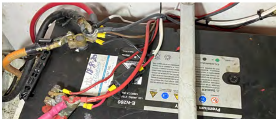
A battery with multiple connections to the terminals. Marine surveyors may be aware that this is not good practice and would recommend a specialist marine electrician be consulted.
