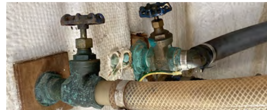
Very corroded seacocks attached to old and brittle reinforced hose. Should either seacock or hose fail, the vessel may experience downflooding. If the bilge pumping system is not spec'd for continuous pumping, water ingress may result in partial or full sinking.
