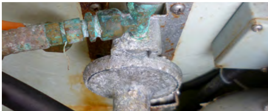
A very corroded regulator and hose for the gas system. This is a good example where surveyors can see a potential problem and advise the owner to seek specialist advice. Gas regulators are generally considered to have a marine service life of approximately 10 years and gas hoses five years.
